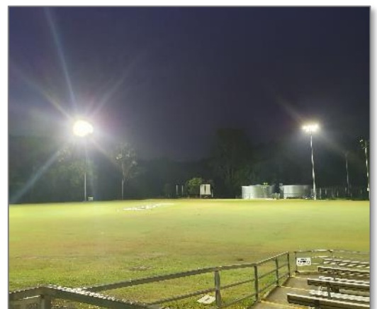
Playing field lighting at Ashgrove Sportsground
